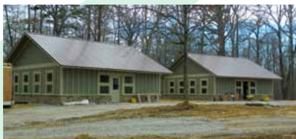
Two new cabins under construction at the J. M Feltner 4-H Camp.
