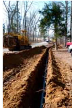
Laying sewer pipe at West KY 4-H Camp, the camp is hooking up to the city system.
